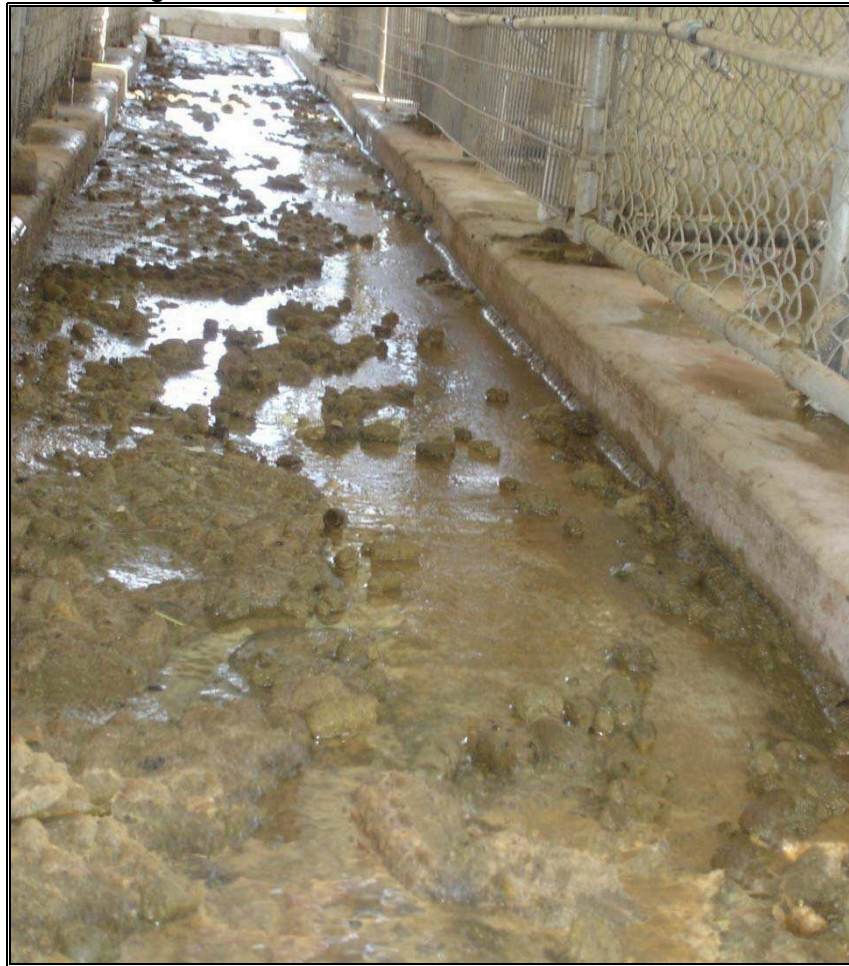
Figure 7: Excessive Accumulation of Feces and Urine
